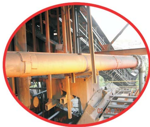
Discarded Traverse Pipe
