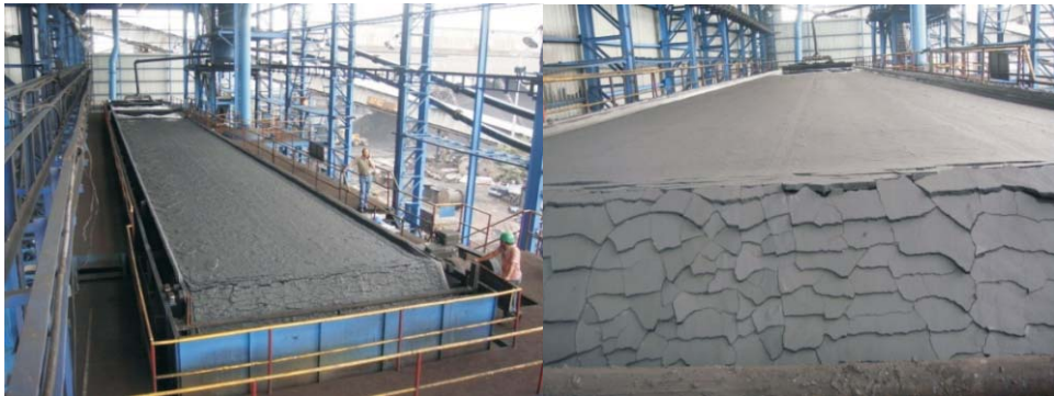
145m 2 Delkor Horizontal Belt filter installation at Washery III West Bokaro, Tata Steel
